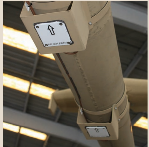
Prototype antenna installation
