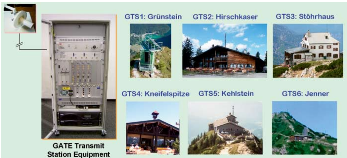
FIGURE 2 GATE Transmitter Locations and Transmitter Rack
