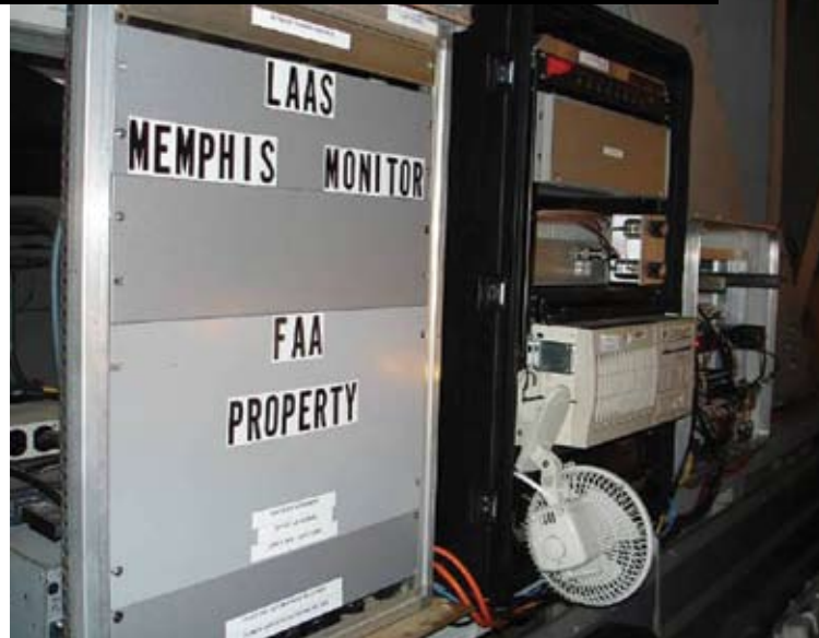
GAEM Installation In Memphis, TN (Photo: courtesy from Tim Martin, FAA)
